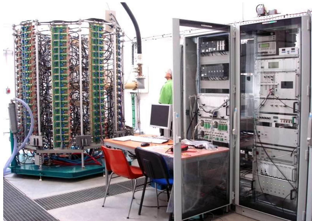
BO RF room (amplifier with LLRF & control)
