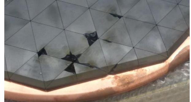
Ferrites are damaged severely.
