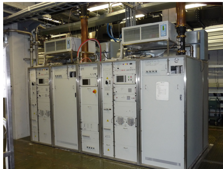
150 kW twin I.O.T.s based transmitter, in operation from 2006
