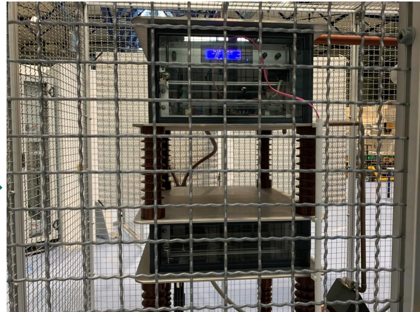
New setup (sector-4) : Power supply + PLC
