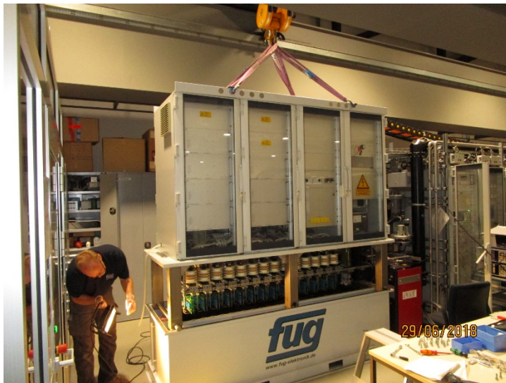
IOT transmitter power supply lifted out of the oil vessel
