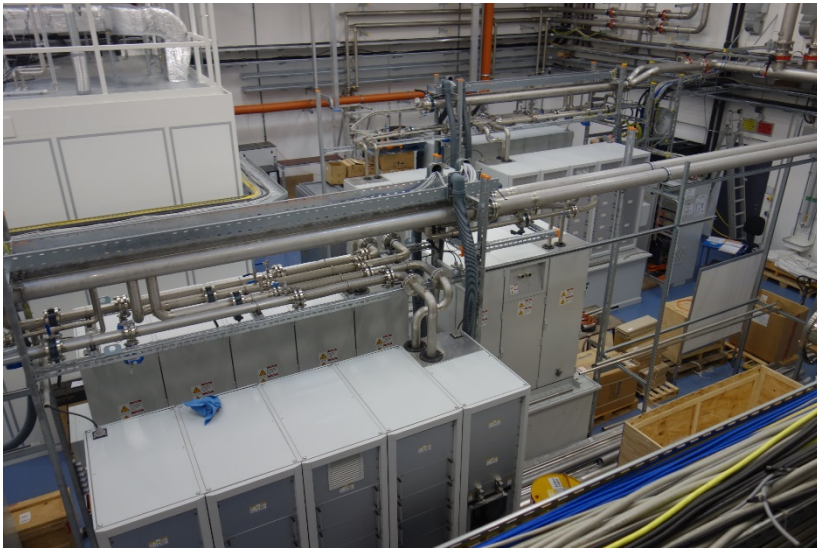
Two 600 kW power supplies
