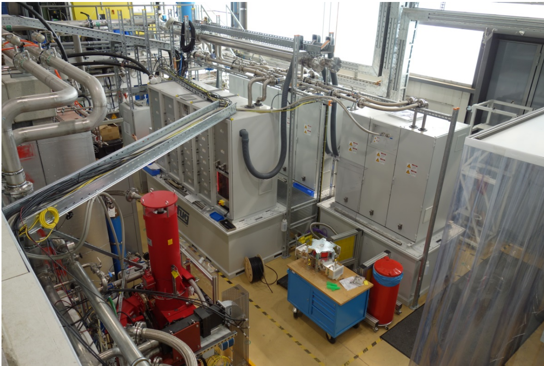
1.3 GHz 270 kW cw transmitter in the testing hall
